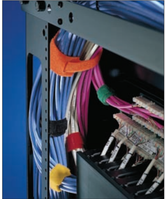
Due to the wide variety of colours available 'One Wrap' ties make cable identification is simple.
